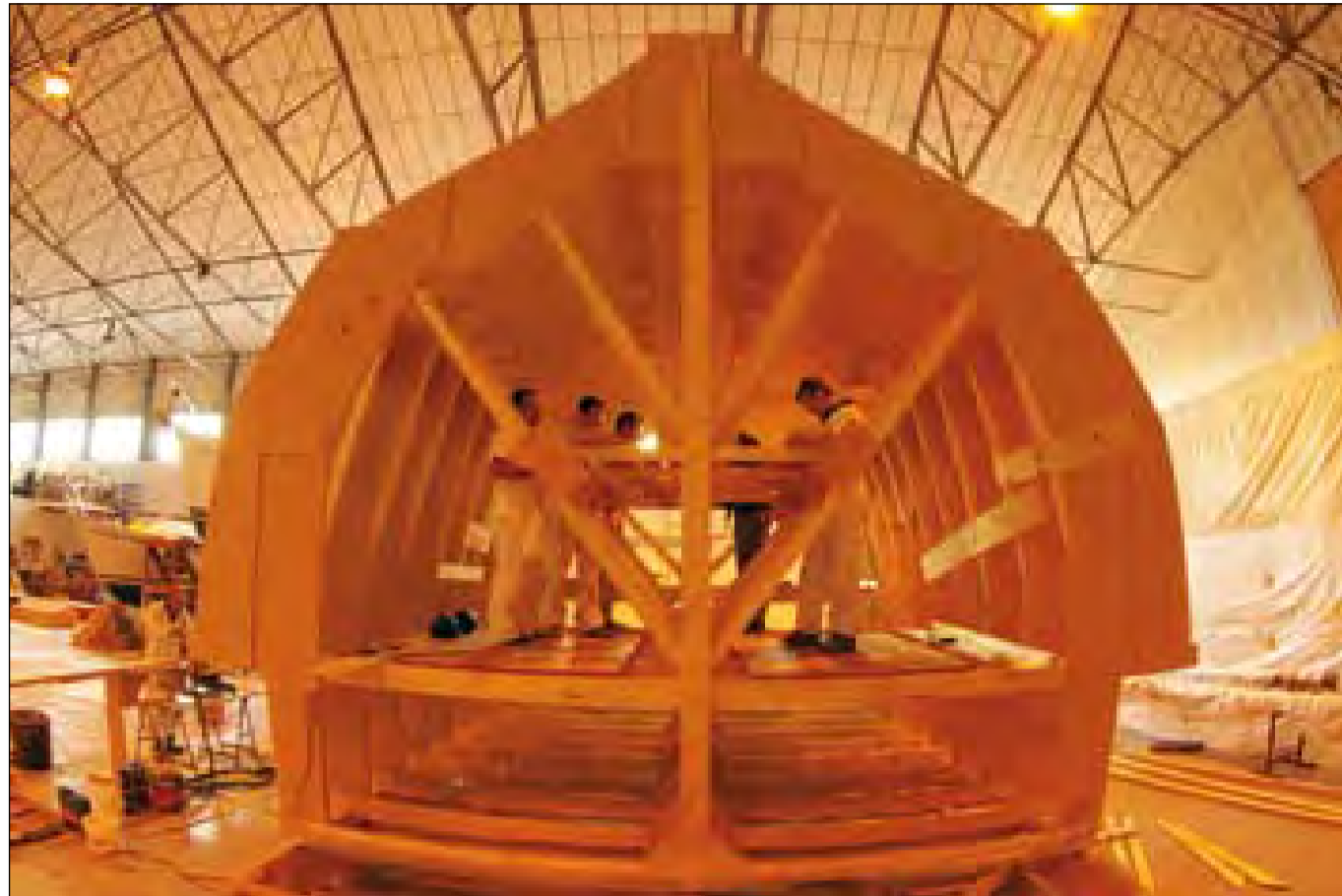
● Work starts on the frame which will be used in the process to create the hull of the TS Jack Petchey
