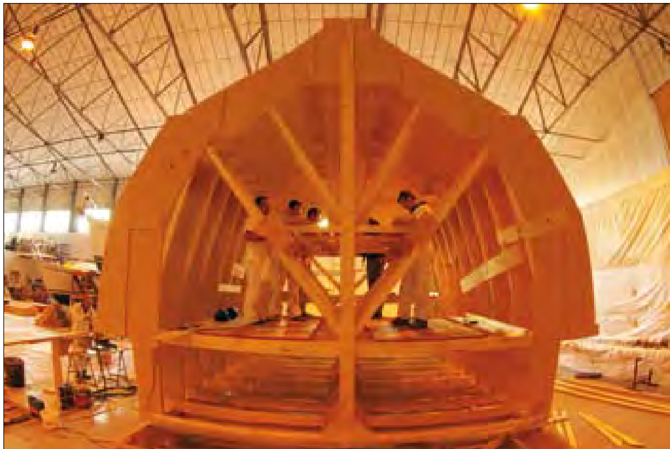
● Work starts on the frame which will be used in the process to create the hull of the TS Jack Petchey
