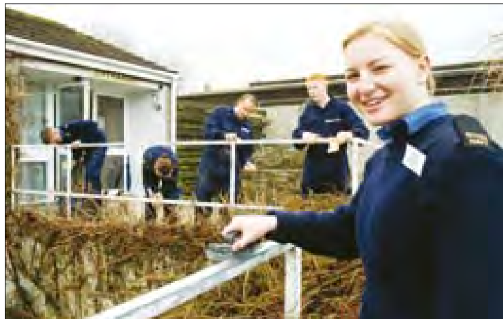
● Trainee Engineering Technician Brooke Wilson and her fellow trainees rub down the paintwork ready for repainting at Pengover Residential Home
