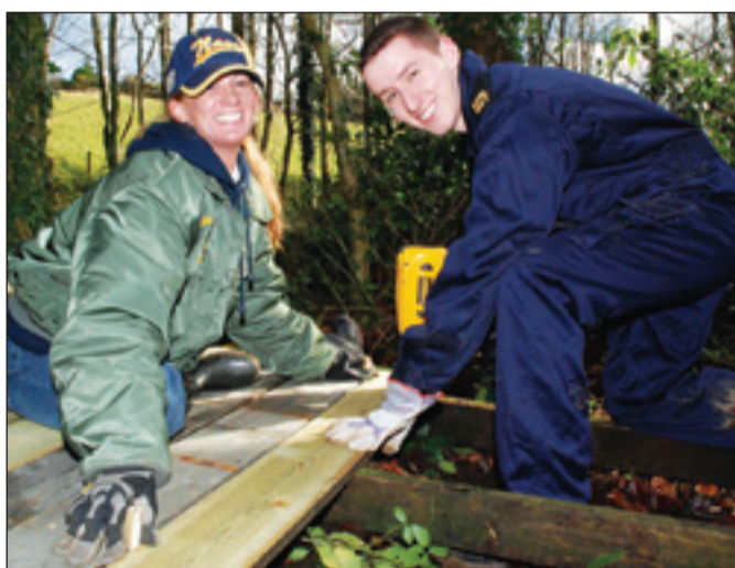
● US Navy and Royal Navy join forces to lay a path at Vitalise Churchtown Centre in Lanlivery
